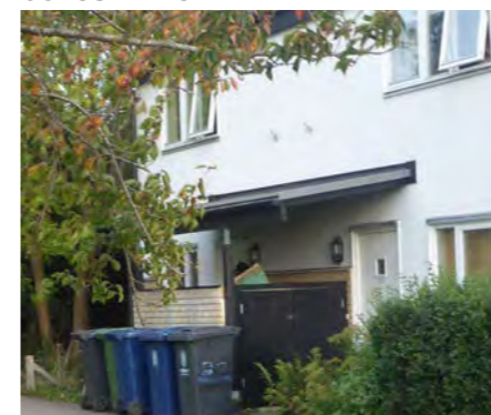
Fig. 88 - Lack of bicycle storage leading to conversion of the bin store
