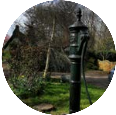
② PUMP TO EAST OF NUMBER 1
