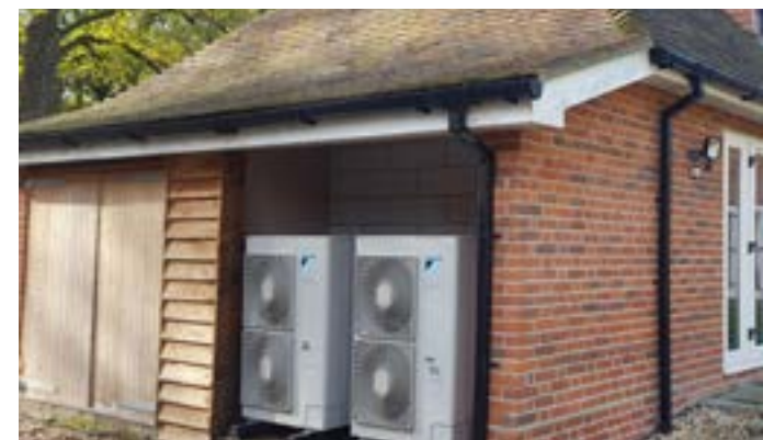
Figure 49: Place pumps in a recessed space to minimise the visual impact
